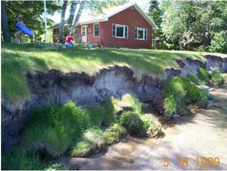
Strawberry Lake Shoreline Repair - Before
