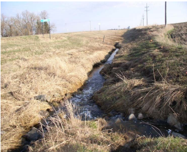
Eroded outlet along highway 59 prior to construction.
