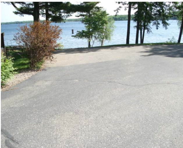
Un-obstructed runoff from impervious surface and surrounding area flowing directly into Island Lake.
