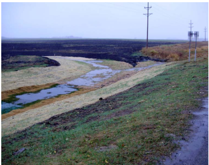
Outlet after construction. This portion was in the Hwy. 59 right of way and was completed by MnDOT.
