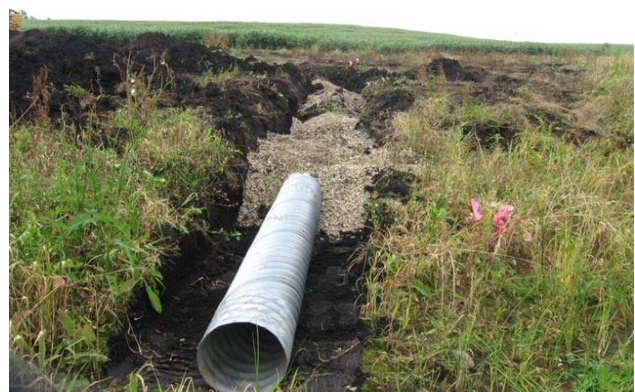
Water and sediment control basin project tile outlet, enveloped in rock before backfilling.
