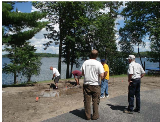
Rain garden is shaped and graded to receive runoff and trap sediments from entering the lake.
