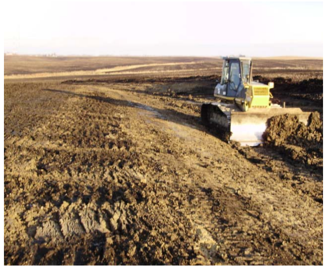
Once tile inlet and basins are completed gullies can be filled in and farmed.
